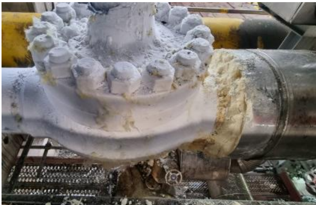
Figure 2. A valve exposed after the incumbent PUR insulation has been cut off Source: Armacell Energy, own photography
